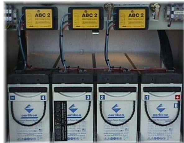
48V Battery system fitted with ABC-2.
